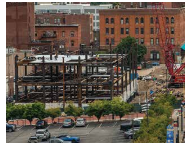
Construction continues on the proposed College of Osteopathic Medicine on Forbes Avenue in Uptown.
